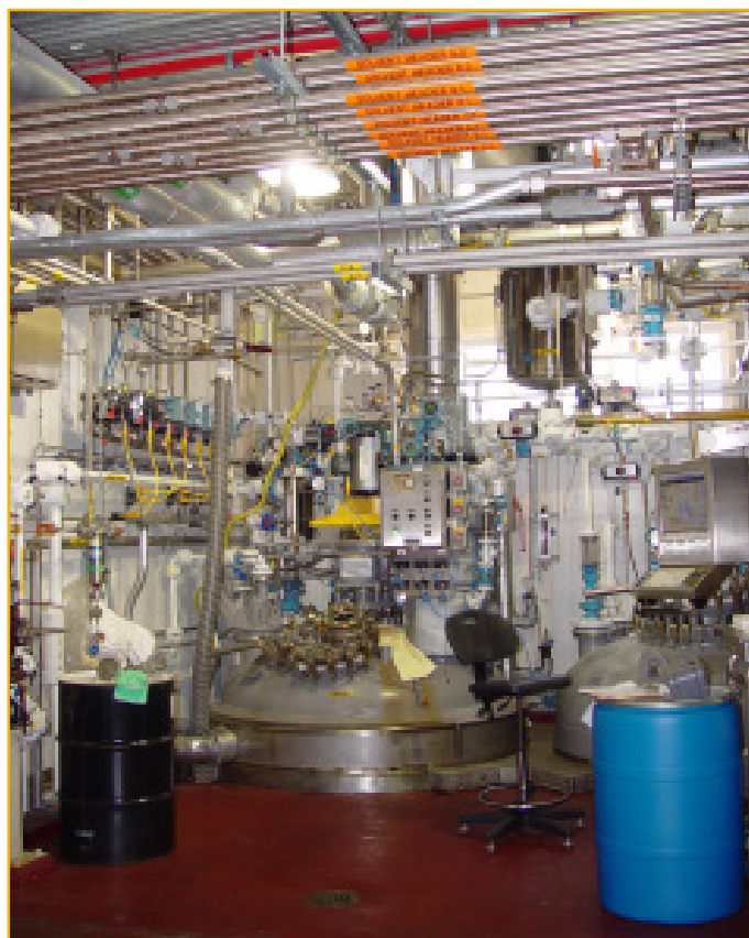
Figure 3. The processing areas are deemed Class 1 Division 1 Group C/D hazardous areas. Instruments can be in Group B/C/D areas.
