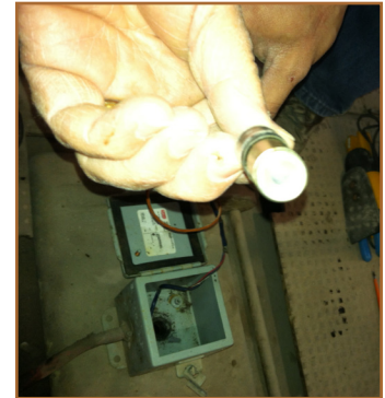
Figure 2. The older, non-contact I/R sensors which had previously been used at the mine. Because they were unable to get close to the ball bearings, they could only measure the ambient temperature near the bearing.
