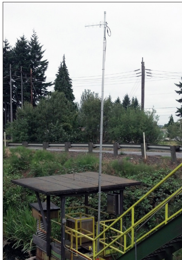
Figure 3. The Yagi-directional antenna was used at the pond site to transmit level signals from the HART level transmitter to the boiler room.
