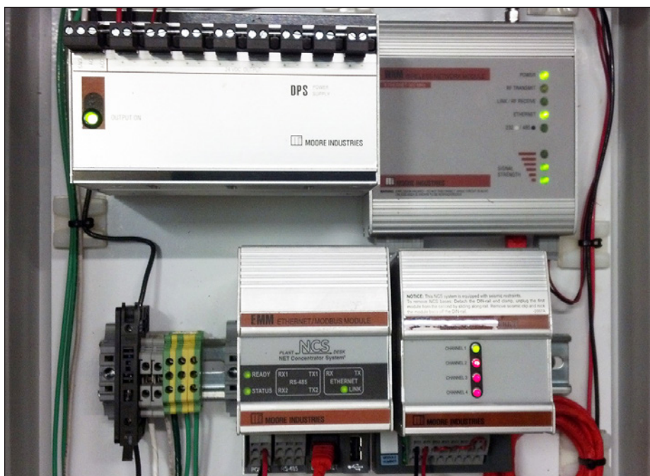
Figure 4. The wireless receiving panel installed at the boiler room of the pulp and paper mill. An Ethernet/MODBUS interface module (EMM) of the NCS serves as a MODBUS master to retrieve HART data from the HCS at the pond site.
