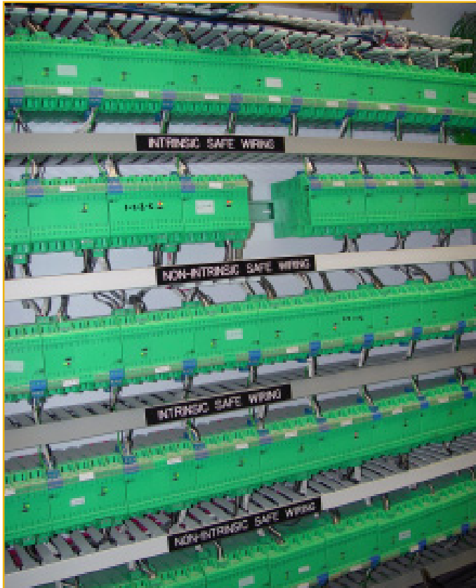
Figure 4. The original ENTITY-based IS system, installed in 2001, required barriers, large cabinets and many fieldbus segments.
